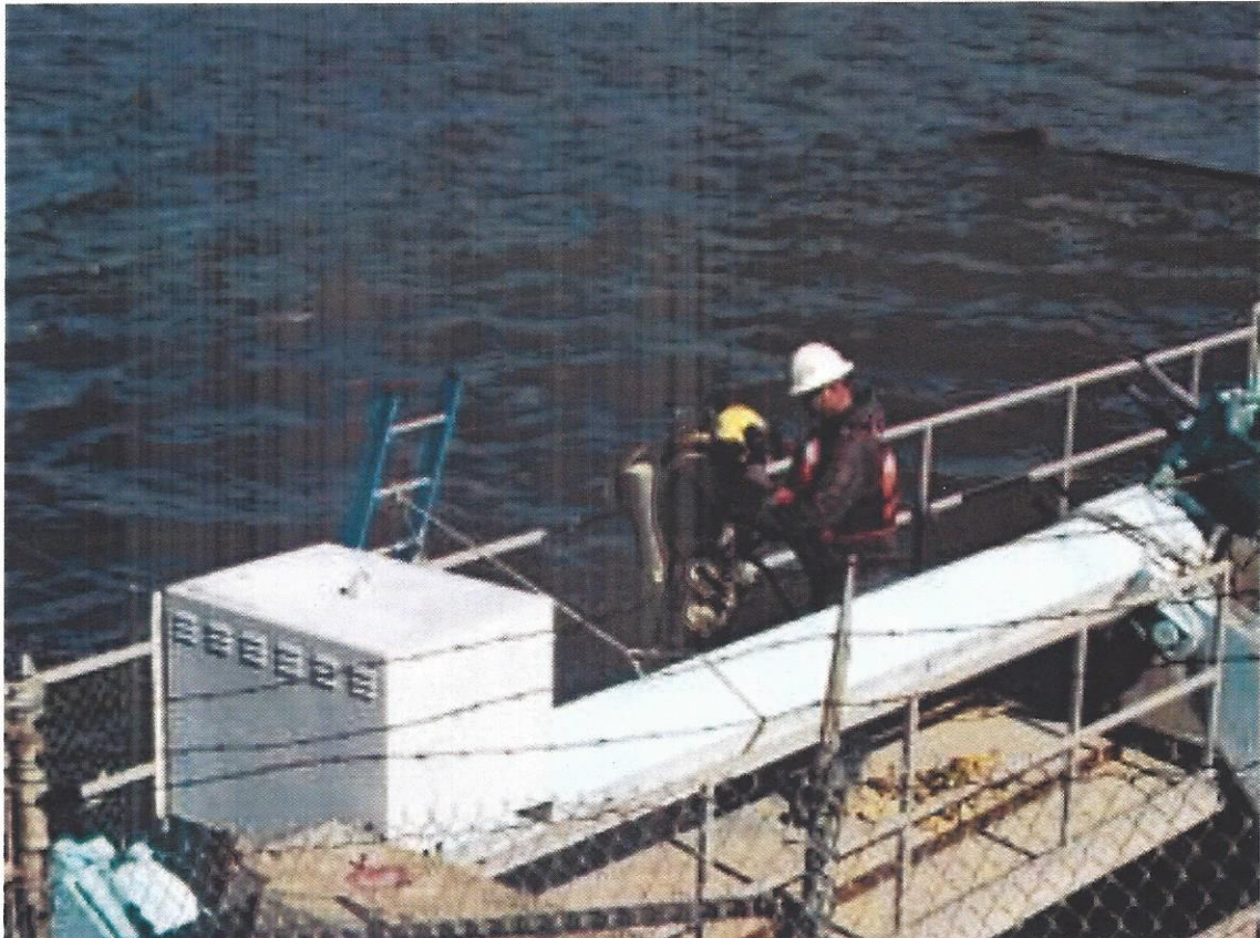
Photo 2: View of the diver getting ready to enter the water from the scaffolding at bay 1.
